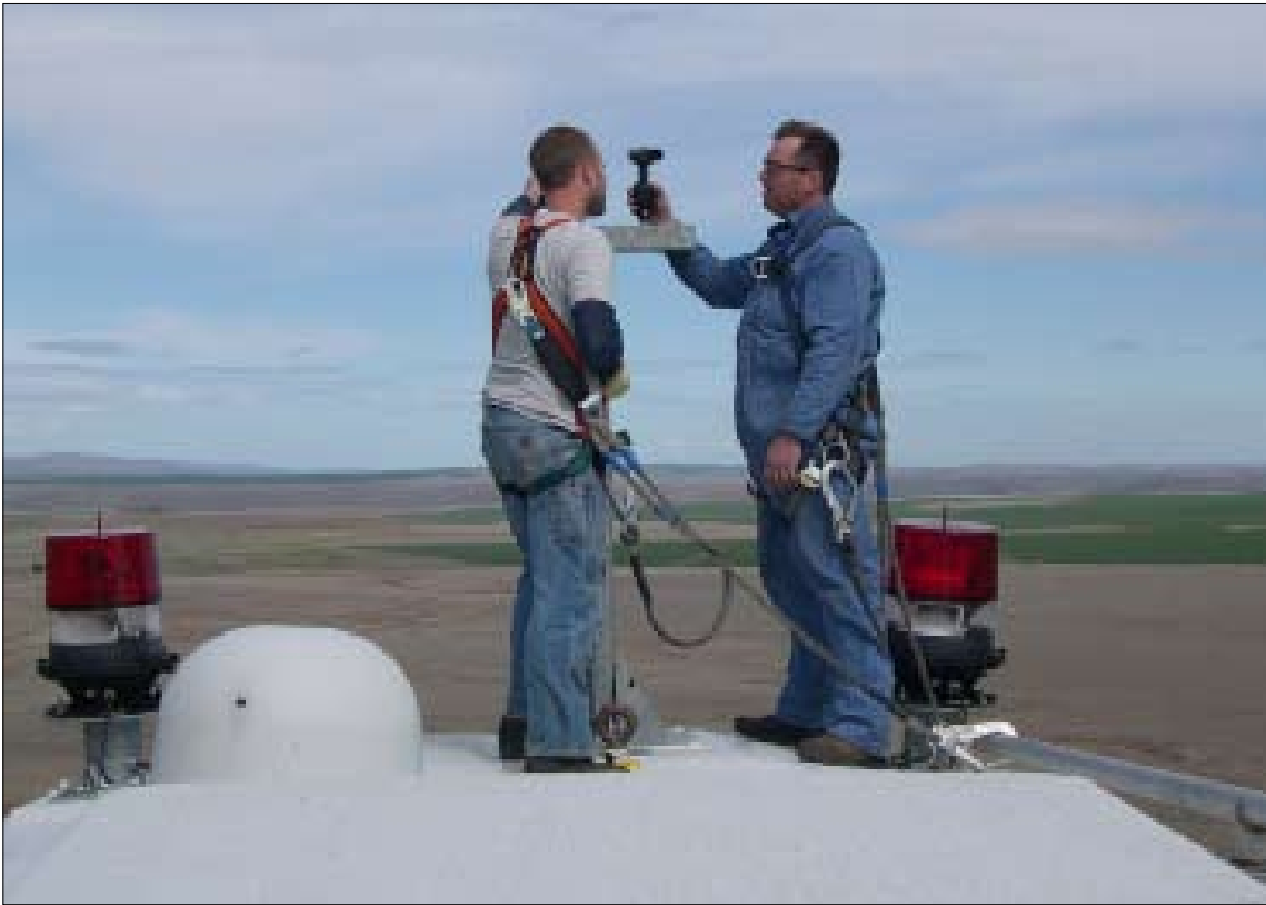
Highflyer: A Columbia Gorge Community College student learns how to work safely on top of a turbine at Klondike Wind Farm
