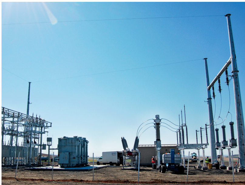
Managing flow Avista's 230kV Boulder transmission substation
